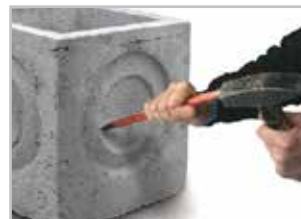
Difficult to open
