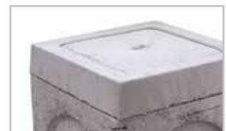
Difficult to open
